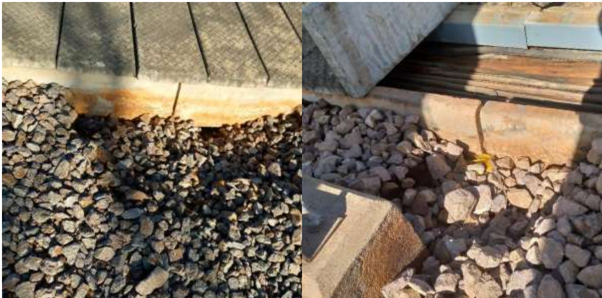
Pictures 8 & 9 – loss of fines and settlements.
