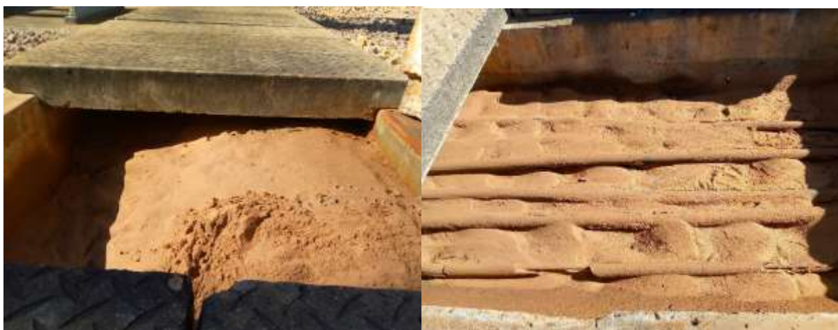
Pictures 1 & 2 – Accumulated material in the cable trench.
