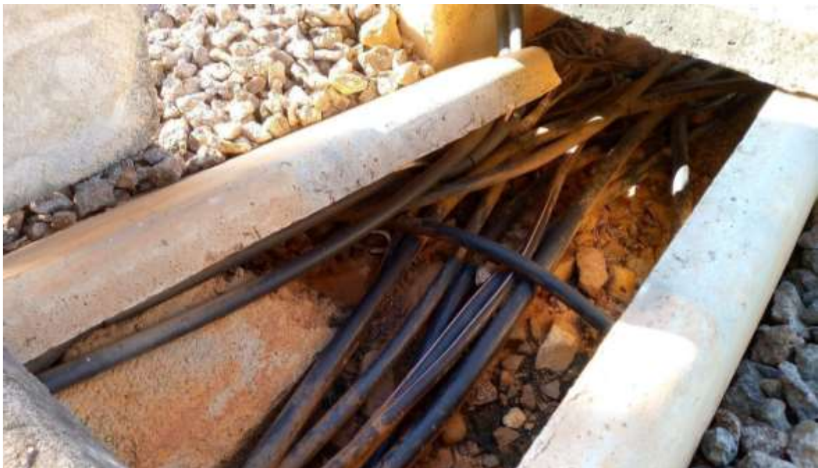
Pictures 3, 4 & 5 – Soils supporting the kerbs eroded, kerb collapsed (Picture 5).
