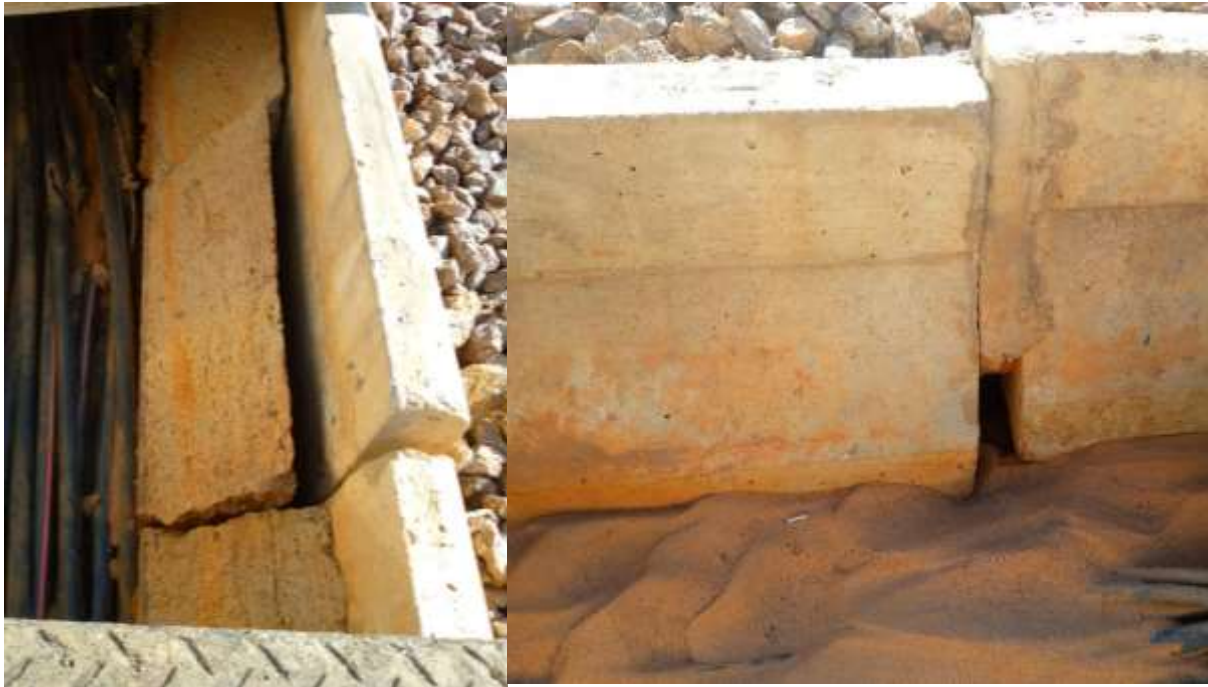
Pictures 6 & 7 – Differential settlement of the kerbs (400 kV zone).
