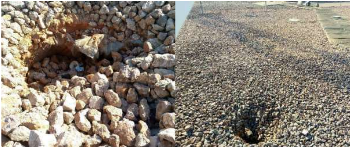
Pictures 14 & 15 – Localised settlement between manholes, 400 kV zone.
