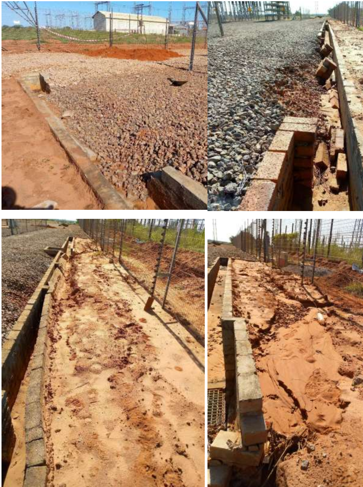
Pictures 16, 17, 18 & 19 – Collapsed walls, intrusion of fines (275 kV Zone).
