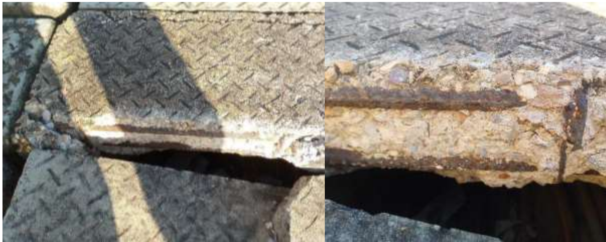
Pictures 10 & 11 – Damaged cable trenches cover slabs.
