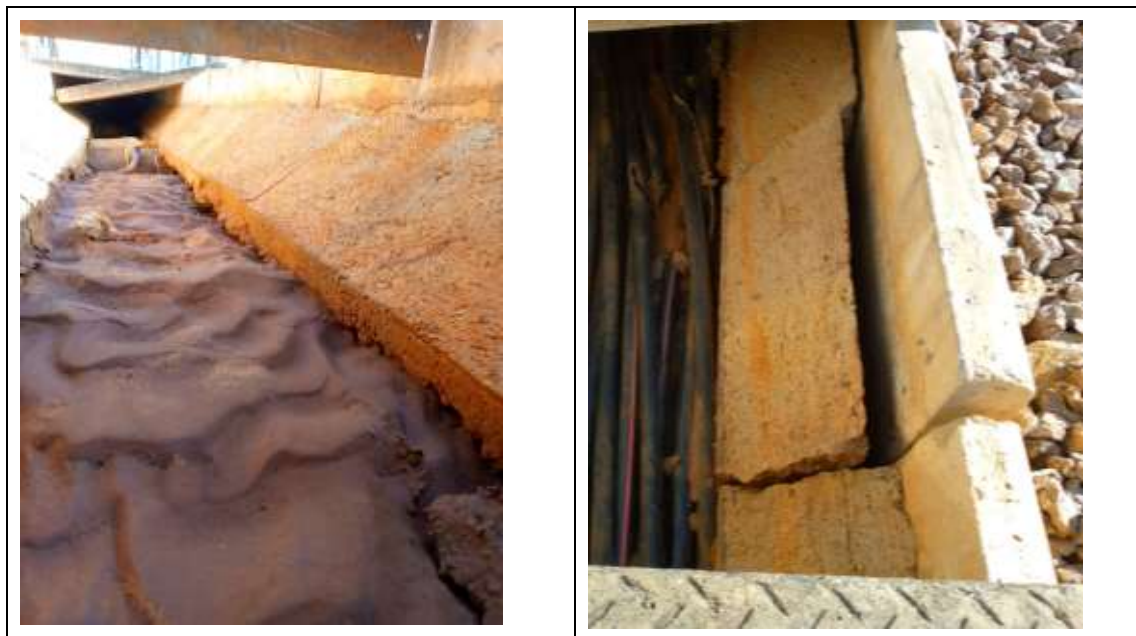
Pictures 12 & 13 – Cables covered with soil and separation between the cast in-situ concrete wedge and the precast concrete kerb (400 kV zone).
